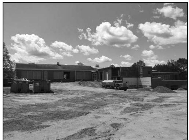
Ray portion removed in preparation for new addition for Town Clerk, Tax Collector and Assessor offices.
